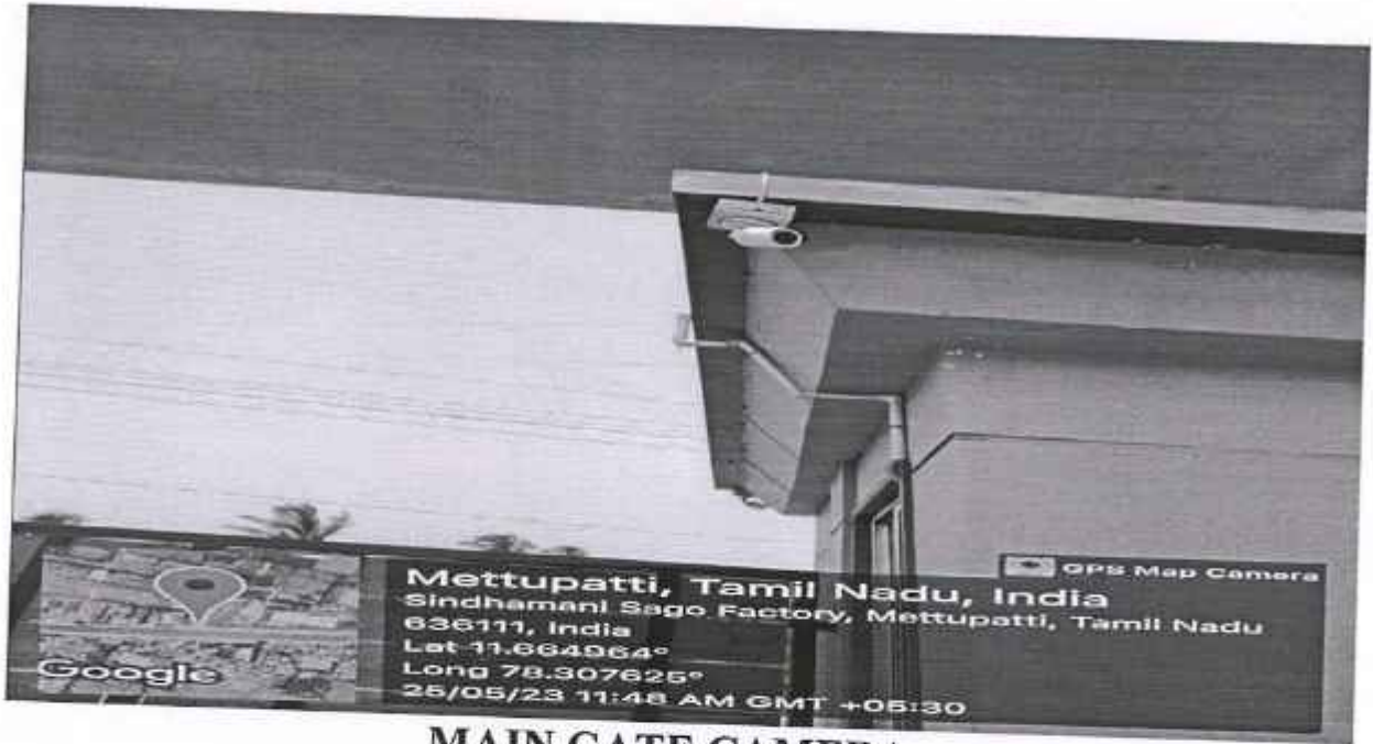
MAIN GATE CAMERA
